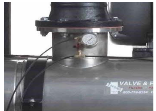
Figure 6: 3-Position manual valve and pressure gauge
